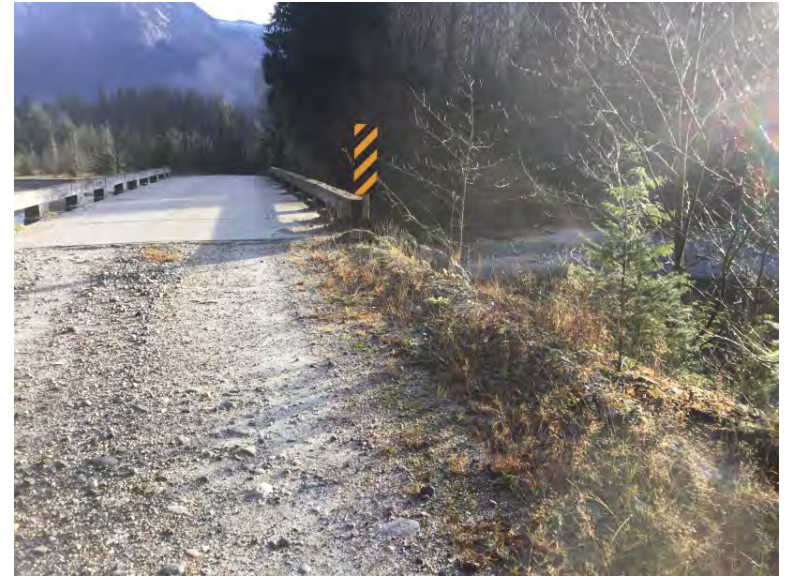
Missing downstream right bank concrete no post barriers
