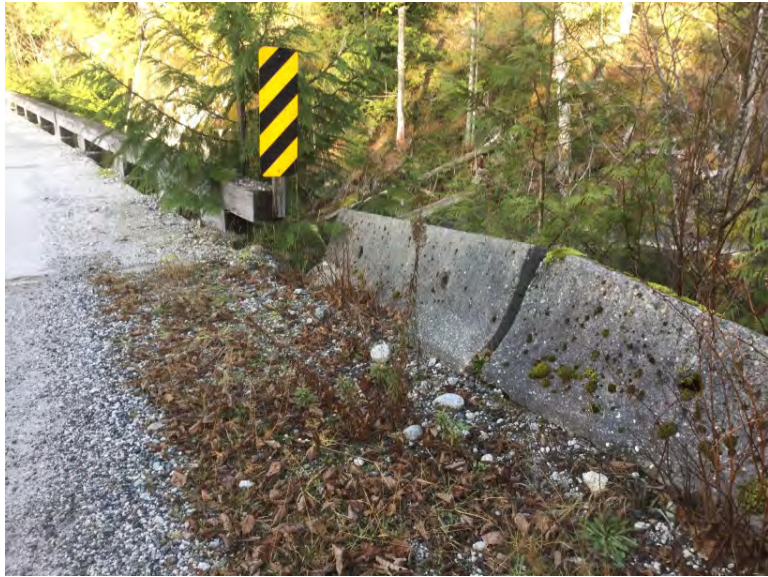
Upstream left approach concrete no posts failing
