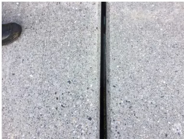
All rubber joint seals failing
