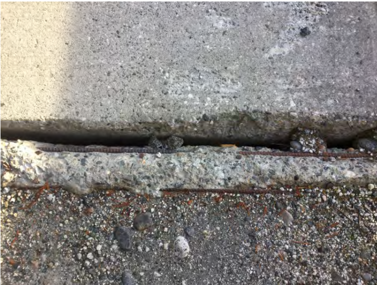
Ballast wall and deck damage
