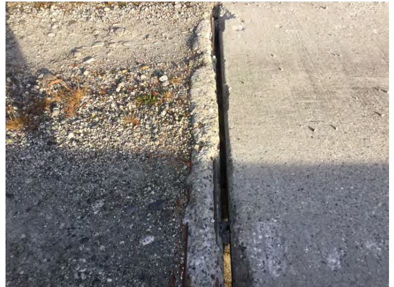
Ballast wall and deck damage
