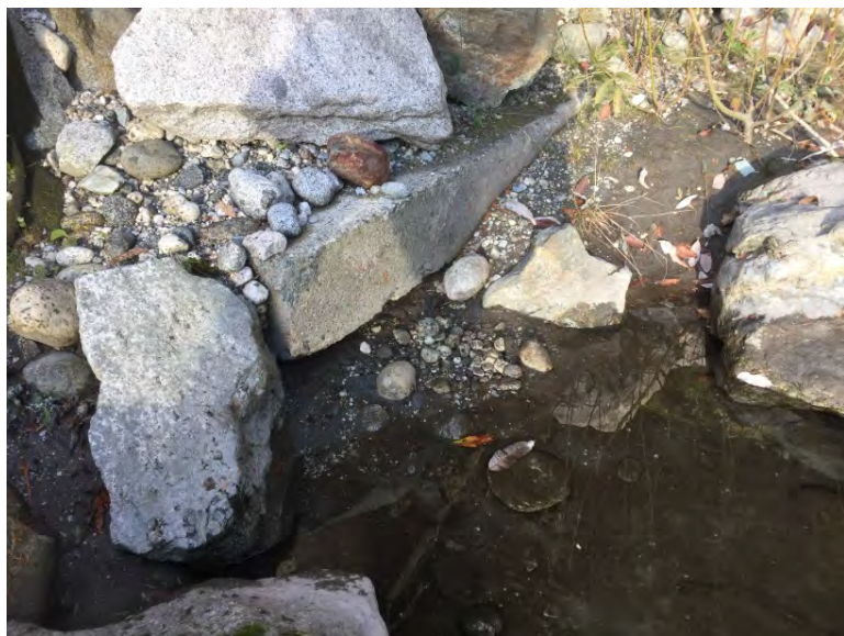
Downstream right bank footing exposed
